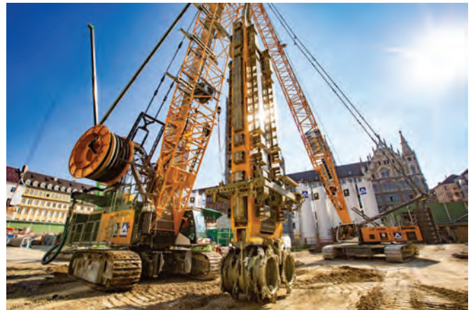
Liebherr LSC 8-18 L slurry wall cutter is currently working on a railway expansion project in Munich. It cuts its way through 33 cu m of soil per hour and requires eight hours for a primary trench.
