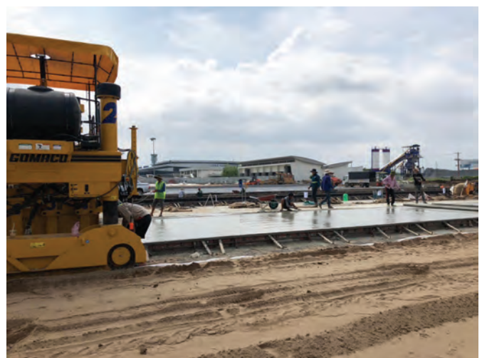
The DKXS 4.00 mixer was running at its maximum capacity of 4 cu m per batch, so that the airport expansion could be finished in the requested time.
