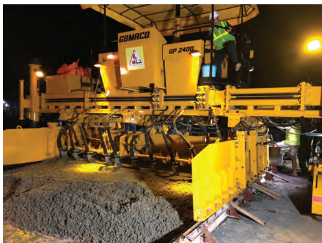
The concrete mixture with big stones of up to 40 mm in diameter was a challenge for the mixing gear.
