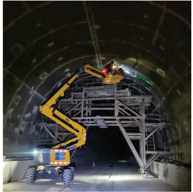
RIGHT: Haulotte HA16 RTJ articulating boom being used in the construction of a section of the Yunnan to Laos railway project.
