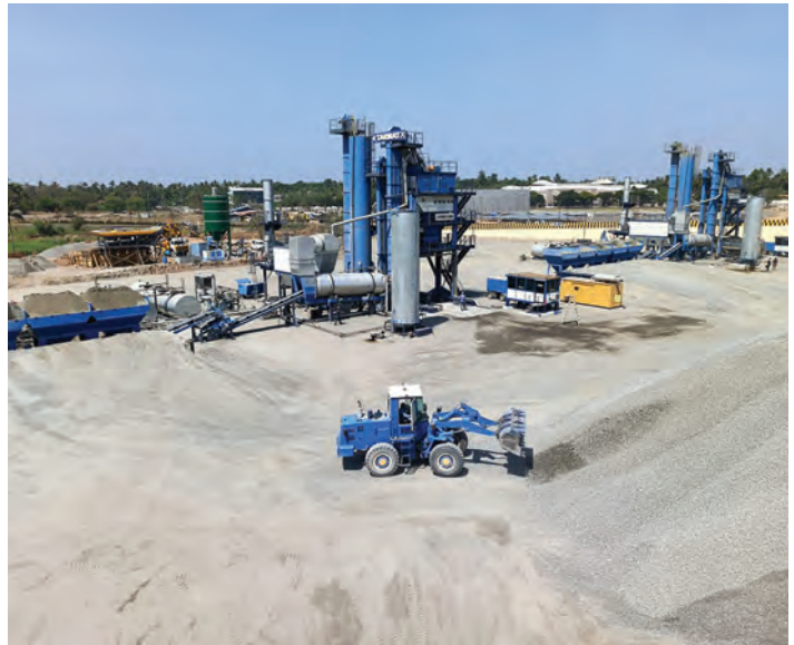
ABOVE AND BOTTOM: Tarmat had to complete the runway project at the Cochin airport within a short timeframe. The job was carried out with the help of Ammann ABC 140 ValueTec asphalt plants and an Ammann sprayer.
